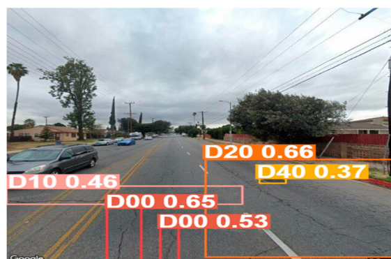
Figure 2: Road damage detected by federated model
